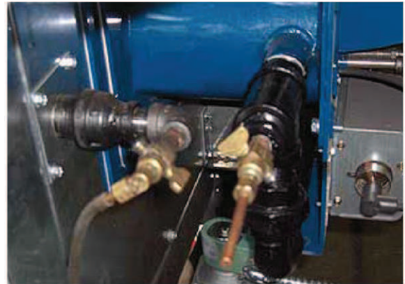
FIGURE 26 - DRAFT OVER FIRE TEST PORT
